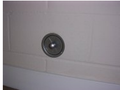
Air vent closed
